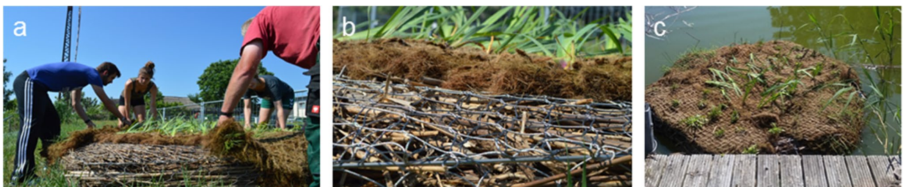
Fig. 1 Installation of first floating wetlands. (A) Pre-cultivated coir mats with macrophytes were placed on the buoyant structure. (B) The carrier consists of an enveloping stainless steel net filled with native dry reed stems. (C) Installation was carried out from a jetty
