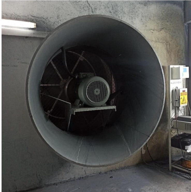
Fig. 1. Indoor Suction Motor in Air Discharge Room
