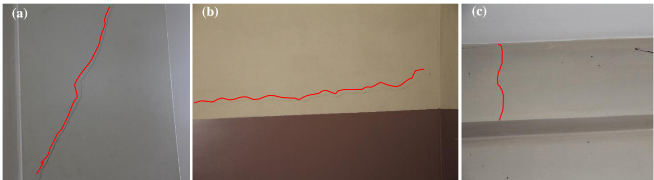
Fig. 6 Damages on the structural elements (a): column; (b): shear wall; (c): beam
