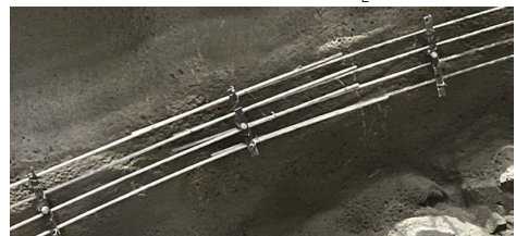
Figure 2 The arrangement of the bars before application of the covering layer of sprayed concrete. T-pieces are used to create an arch
