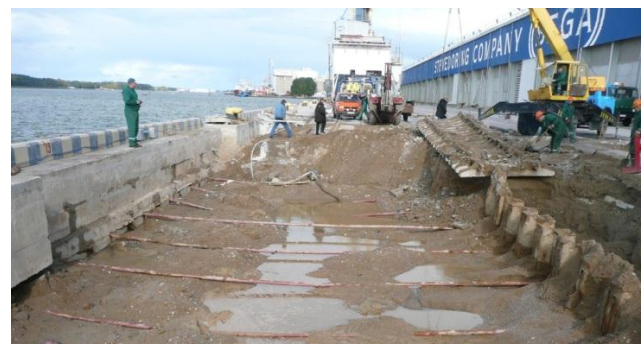
Fig. 9 Real situation of quay wall with anchors and VHP columns (after excavation)
