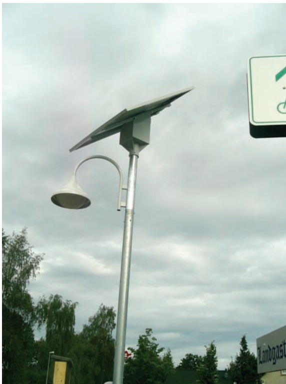
Solar-LED luminaire in Berghausen as self sufficient installation – Leuchten GmbH, Pasewalk, 28 W, 3.400° K.
