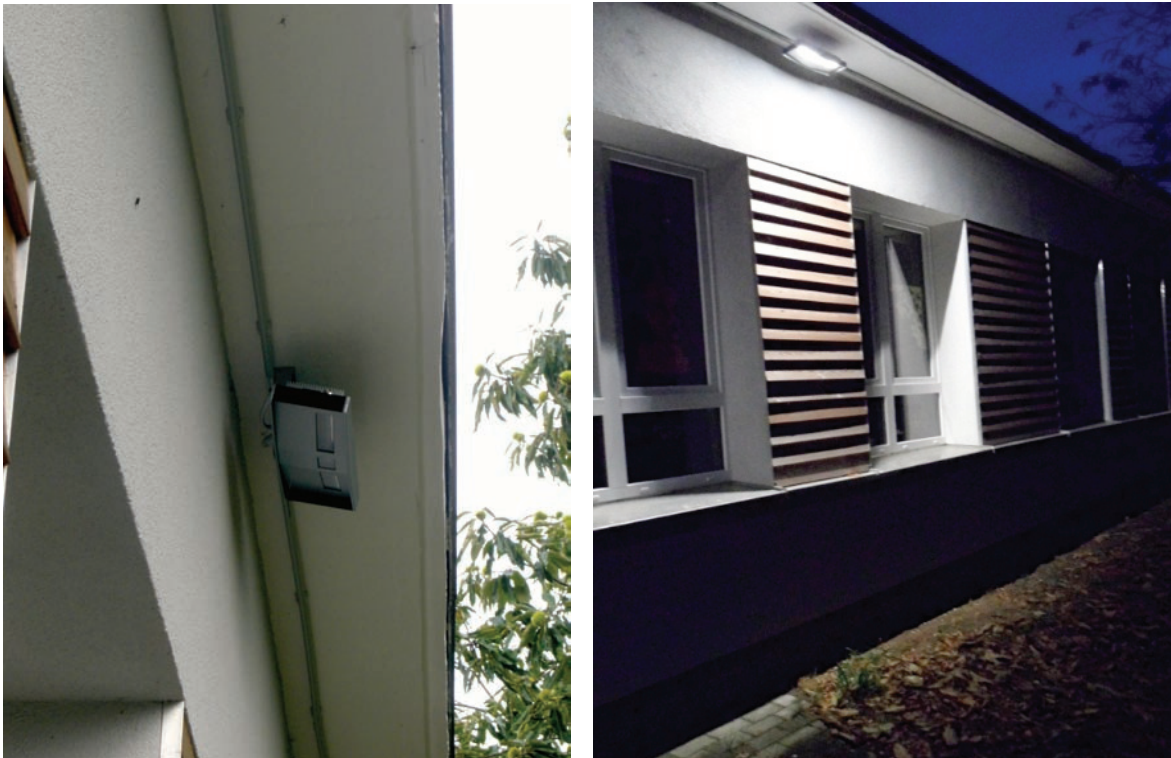
Façade lighting - 4 x Sill spots, 18 W, 3.000 K, dimmable.
