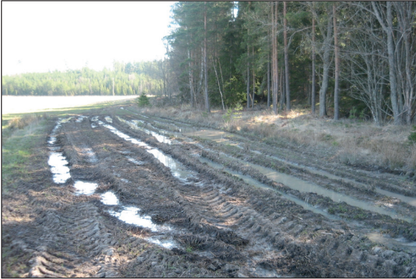
Figure 9.10. Missing ditch and poor drainage in the county of Östergötland, SE Sweden. Photo: B. Ulén.
