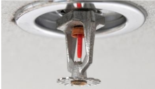
Picture 7. Automatic fire extinguishing systems – sprinklers 439
